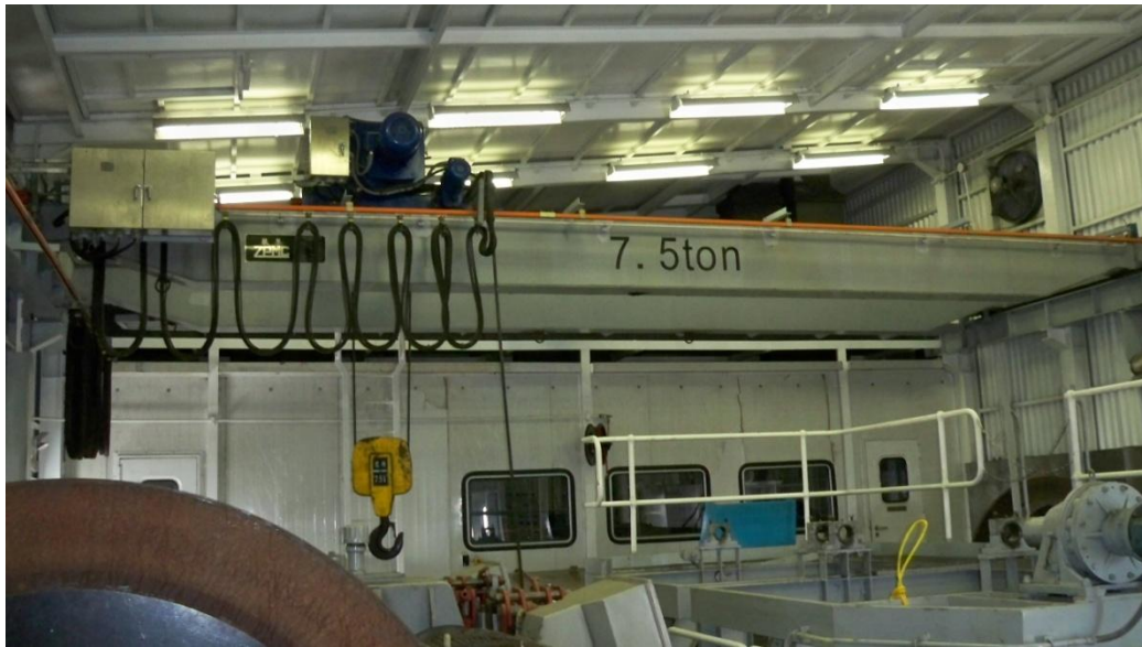
Machinery House Service Crane
