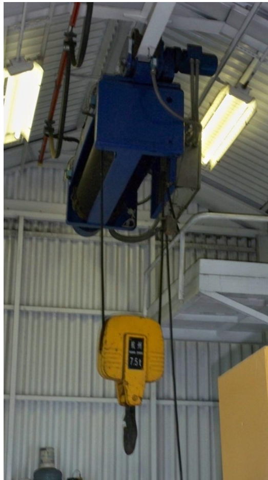
Generator House Service Crane
